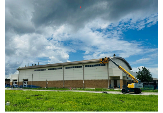
OPSB Lake Forest Cost $1,333,501 School Renovation after hurricane Damages
